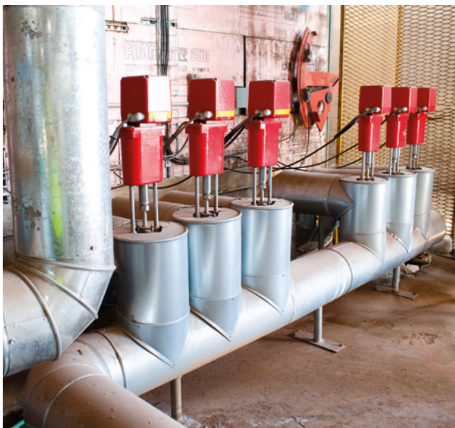
Kraft Curing Vapor Control Valves to Control Temperature in each Chamber
