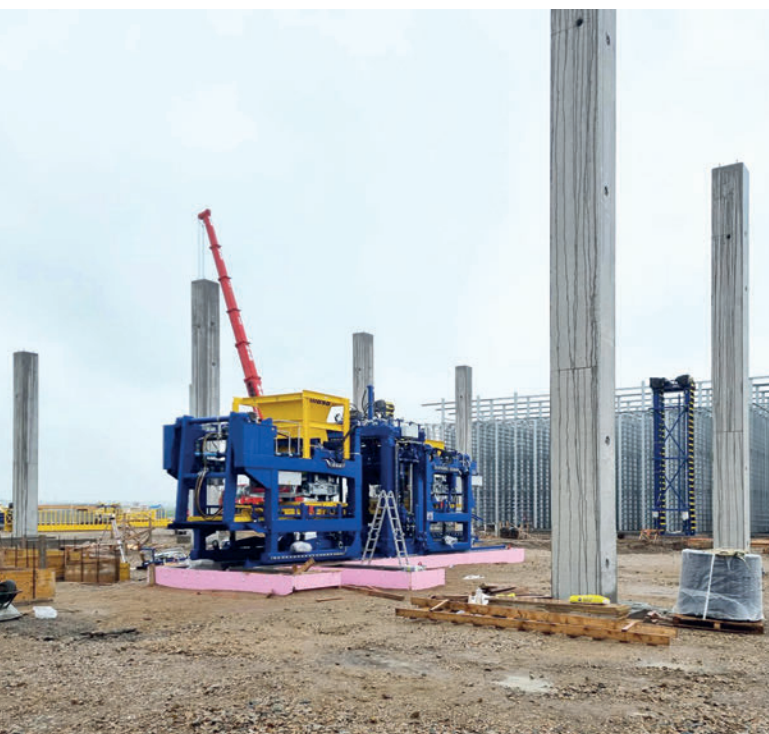
Early stage of construction: Step by step, the new high-tech plant is being installed around the Masa XL-R.
