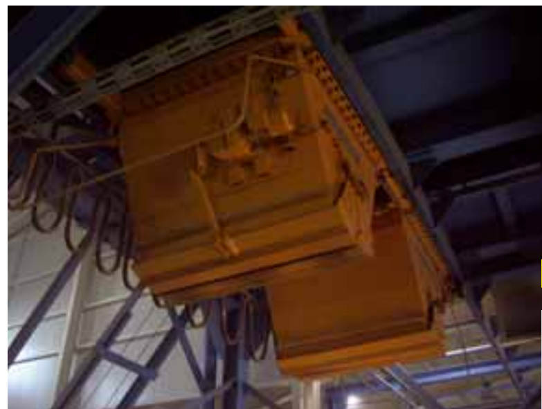
Bucket conveyor system
