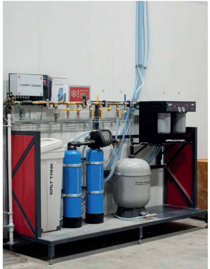
The Genest installation incorporates Kraft's AutoFog moisture addition system.
