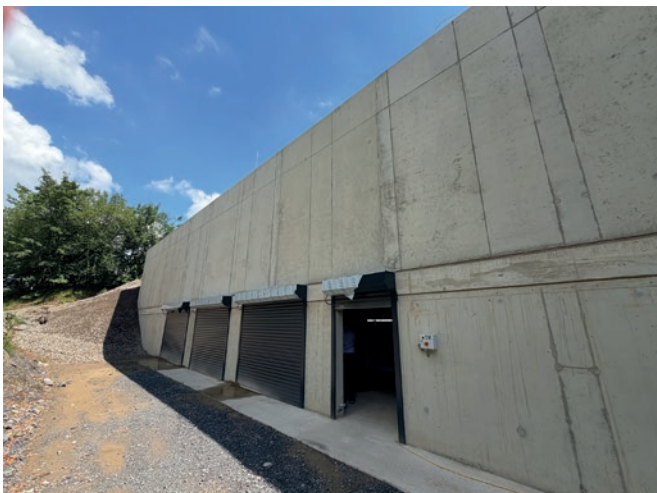
The aggregates are stored in 7 inline aggregate bins that are embedded into the foundation and have a total volume of approx. 400 m³.
