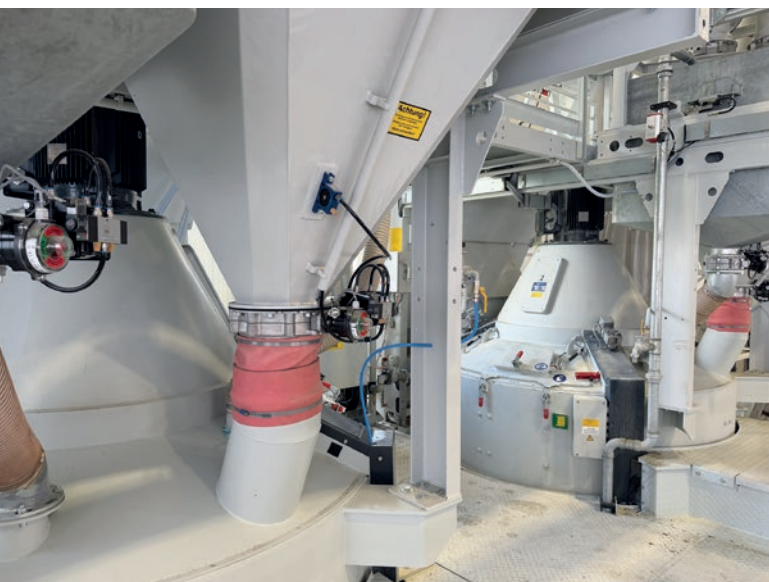
The core elements of the newly installed double-mixing plant are the two Wiggert planetary mixers of type HPGM 1875.
