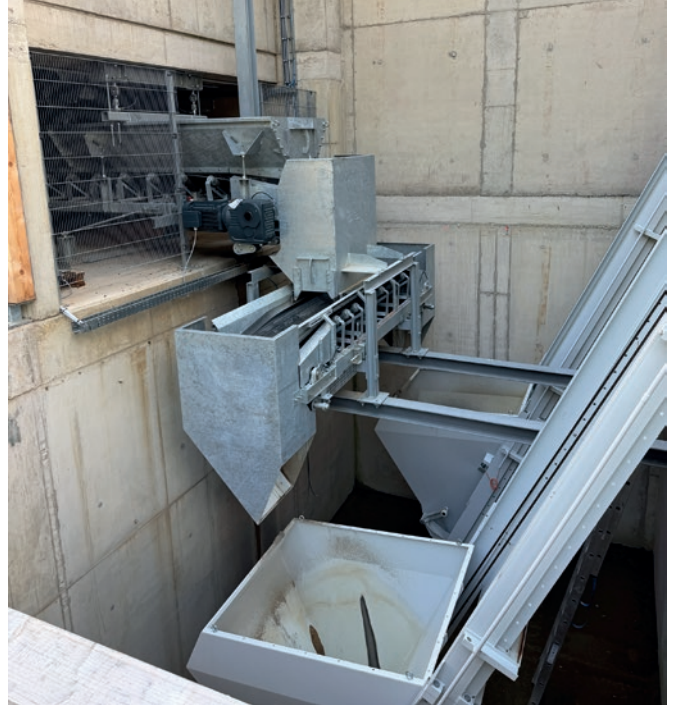
Depending on the direction of belt travel, the distribution belt fills one of the two skip hoists.
