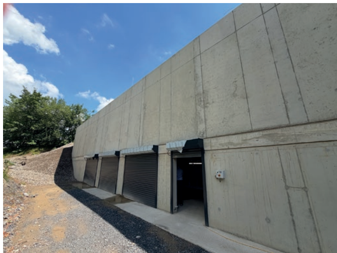
The aggregates are stored in 7 inline aggregate bins that are embedded into the foundation and have a total volume of approx. 400 m 3 .
