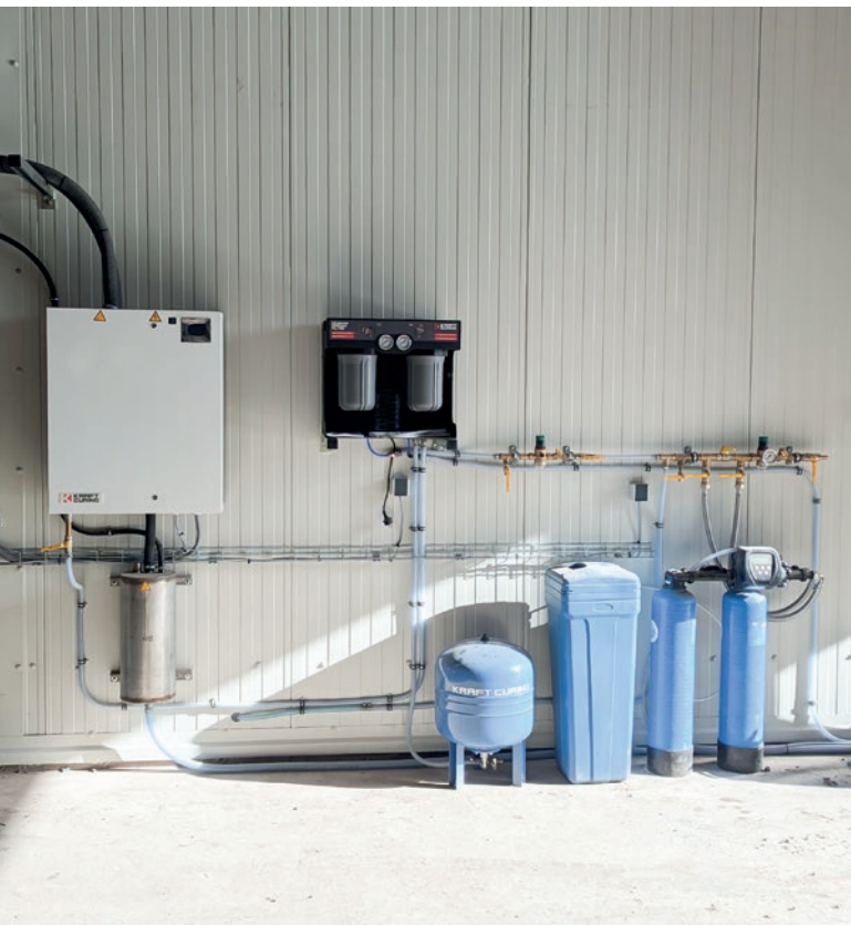
To regulate humidity precisely, Kraft integrated its AutoFog moisture addition system into the curing chamber.
