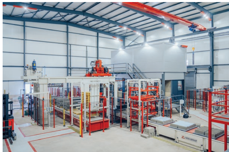
In defined cycles, the boards move beneath the block and paver splitter, which precisely pushes products together and aligns them for downstream processes.
