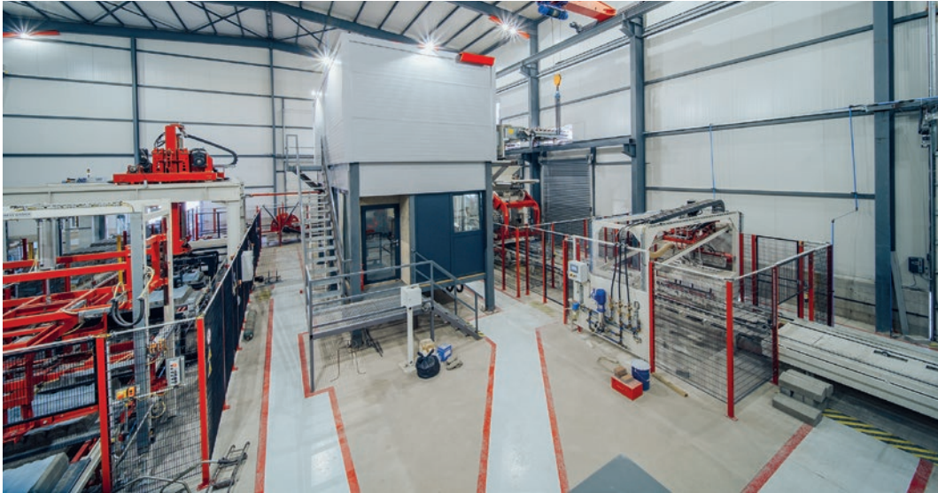
Overview of the wet and dry sides
