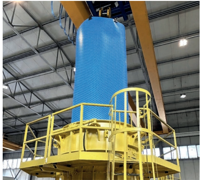
Inserting the liner cylinder made from Agru concrete protective liners into the 4 m-high pipe wetcast moulds
