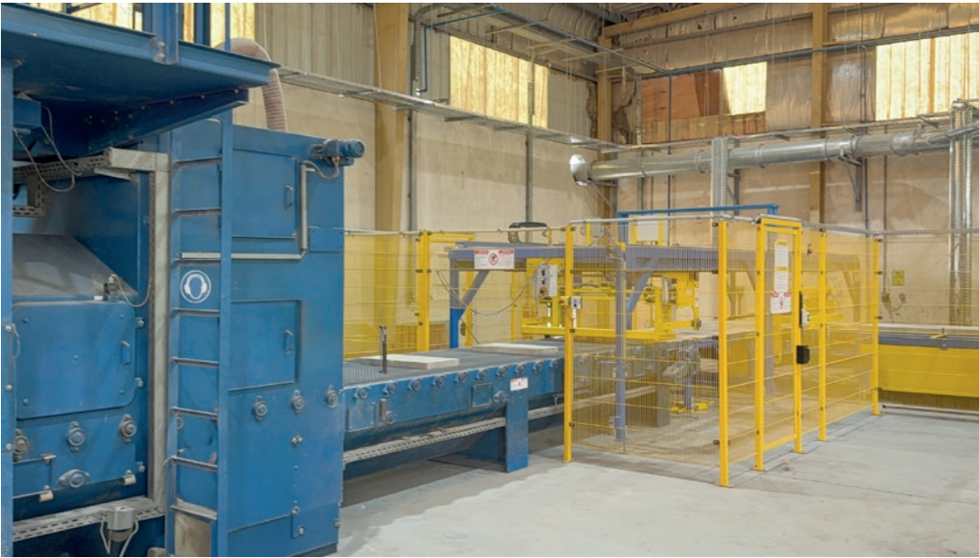
Existing shotblasting machine - provided on the construction side and integrated into the facility
