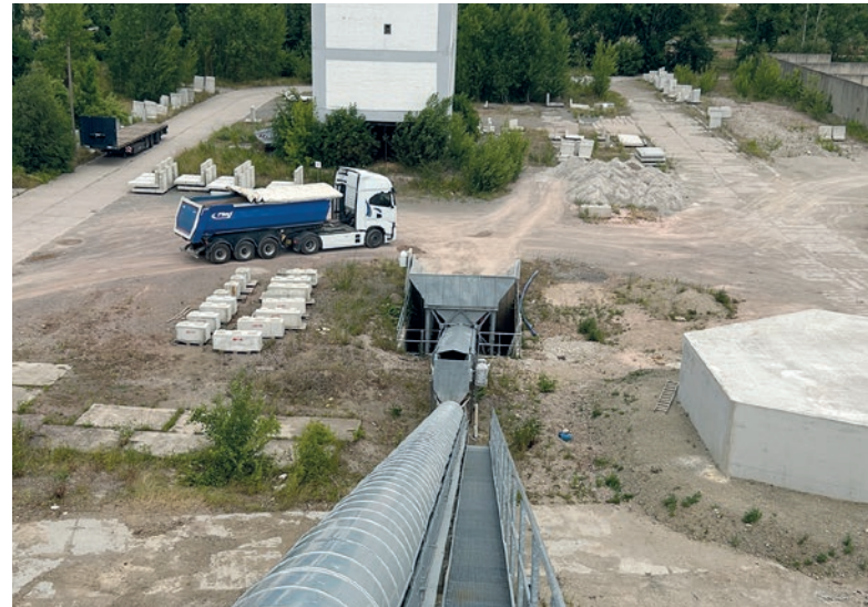
The 6-chamber in-line silo is fed via a flat feed hopper (complete lorry load) and a belt system.
