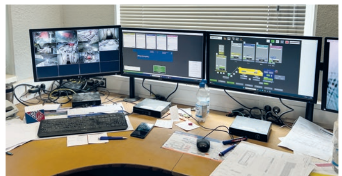
Control room of the mixing plant
