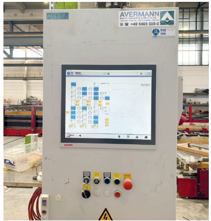
Together with RIB One Prefab Automation and Avermann, a customised HMI/SCADA system with intuitive touch operation was created.
