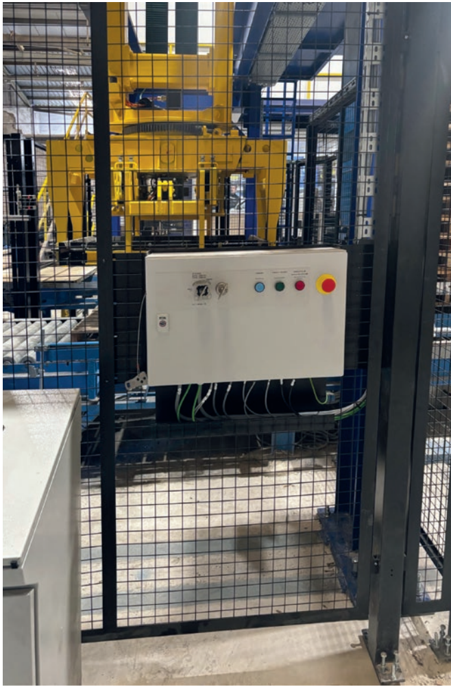
The Masa Safety Concept – reliable protection for operating personnel with very high system availability
