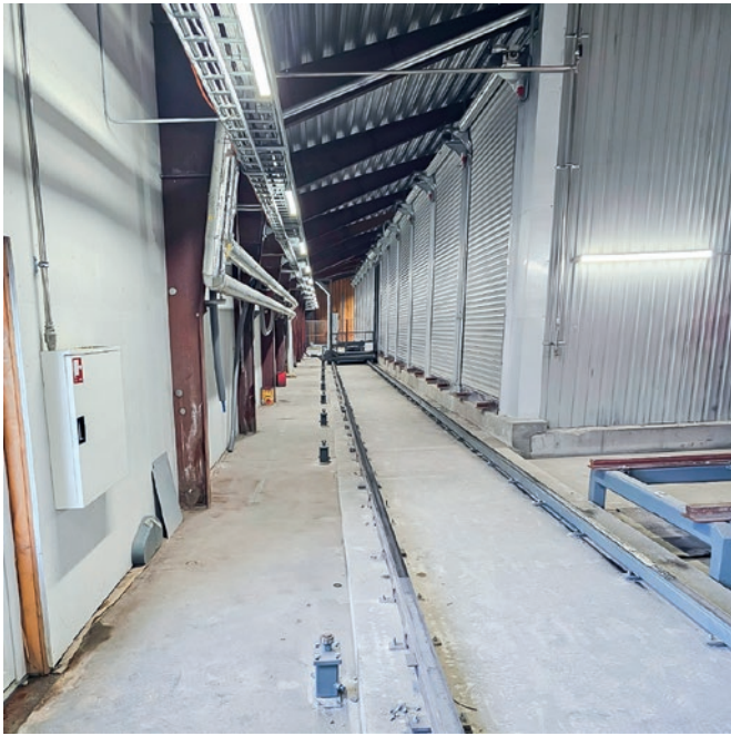
The 13 new FIFO curing chambers with insulated motorised aluminium roller doors
