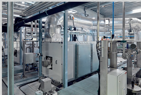
Successfully installed plant
