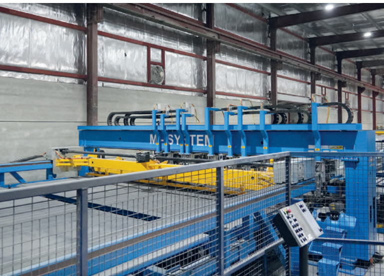
The M-System mesh welding plant is fully automated and saves a lot of time and manpower.
