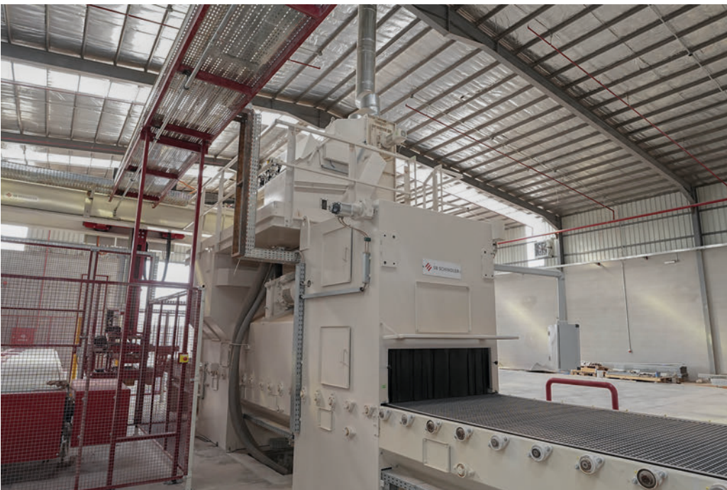
Shotblasting unit (in commissioning)
