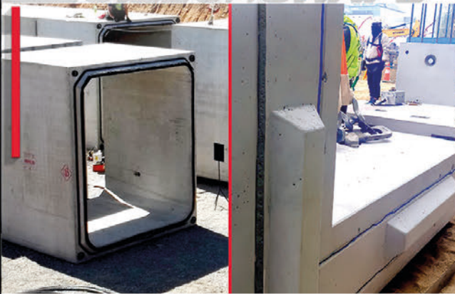
1 MILLION GALLON WATERTIGHT STORMWATER DETENTION SYSTEM
