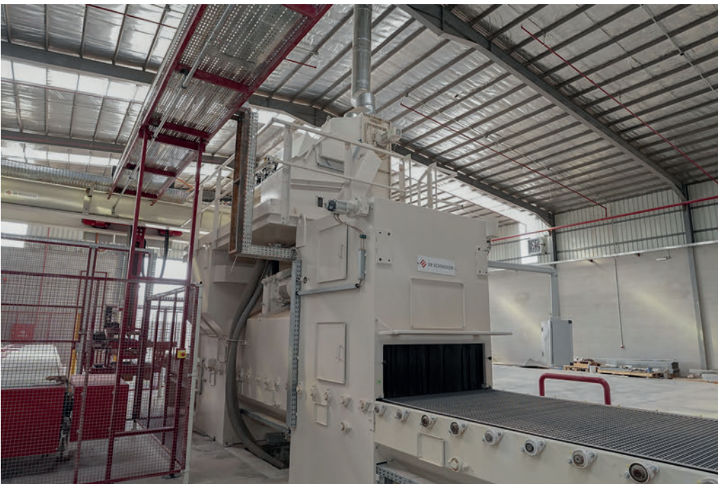
Shotblasting unit (in commissioning)
