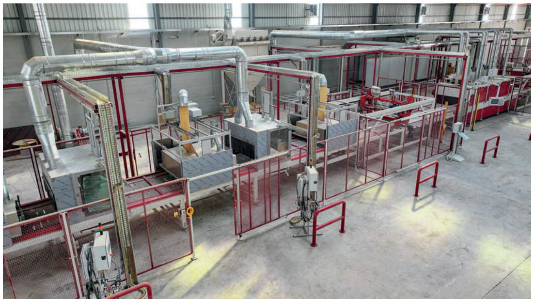
Coating line (in commissioning)
