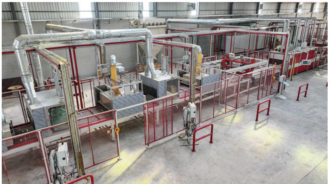
Coating line (in commissioning)
