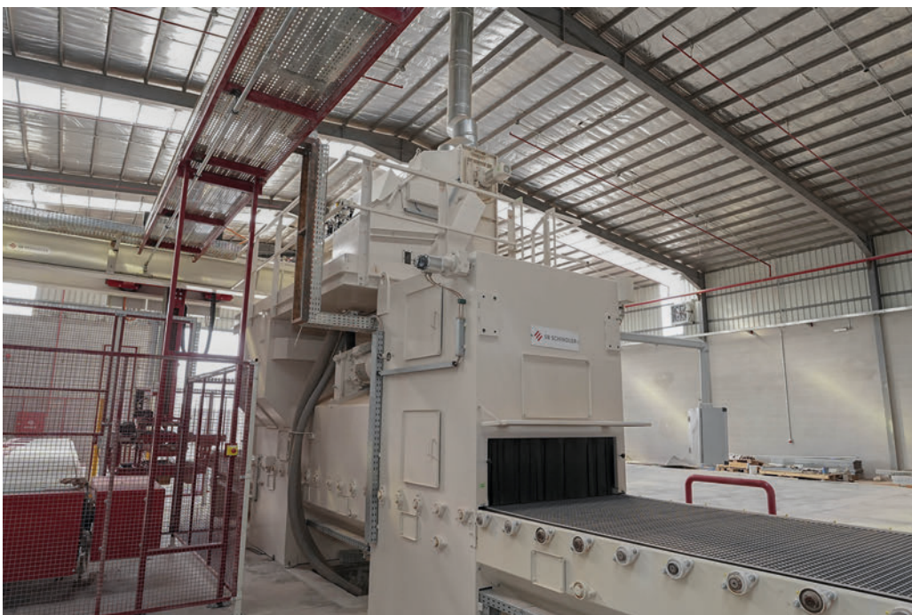
Shotblasting unit (in commissioning)
