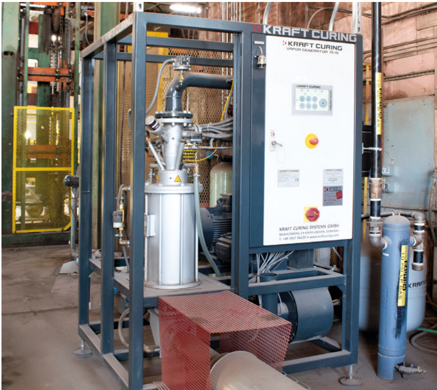
Kraft Vapor Generator 15-1S Replaces Old Boiler System
