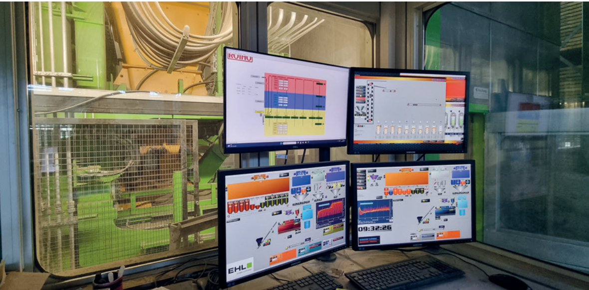
Centralised control of the dosing and mixing plant via the Sauter s-mix process control system.
