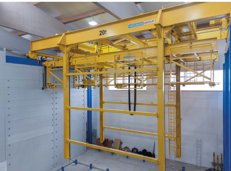
The storage and retrieval machine stores the pallets with the freshly concreted elements in the drying chamber, which now enables the precast concrete elements to cure efficiently.
