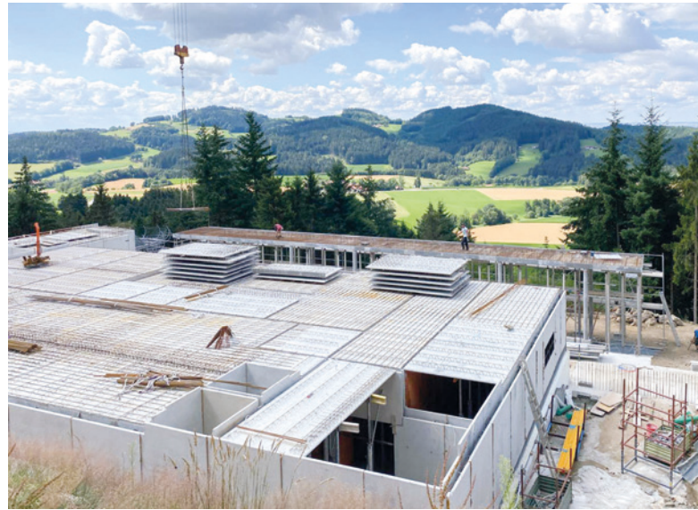
The mountain inn in the Edelwies leisure park in the Bavarian Forest is currently being built with the precast elements from the new factory.
