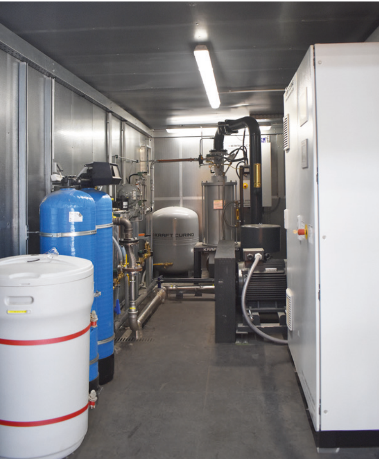
The Containerized Vapor Curing Unit with Water Treatment System.
