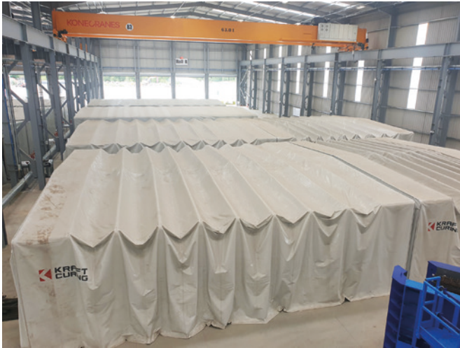
Some of the many retractable enclosures inside the secondary curing area. Each enclosure is capable of containing two concrete elements.
