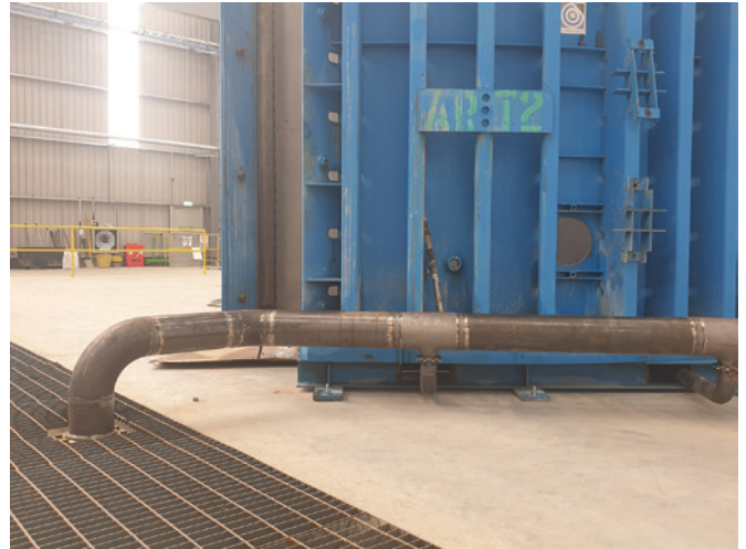
Primary Curing in the Permanent Facility - Pipe trenches keep the production floor free from obstructions. The vapor is always delivered at ground level, directly under the form for best temperature consistency.
