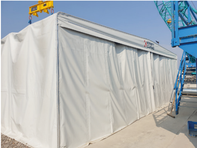
One of the five retractable curing enclosures (tents) initially supplied to the outdoor temporary casting area. The tents could be quickly dismantled and moved to the permanent facility once completed. A further ten tents were supplied as part of phase 2 delivery.
