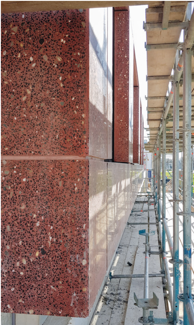
Facade elements by Preco at the construction of the hotel "The bridge" in Amsterdam.
