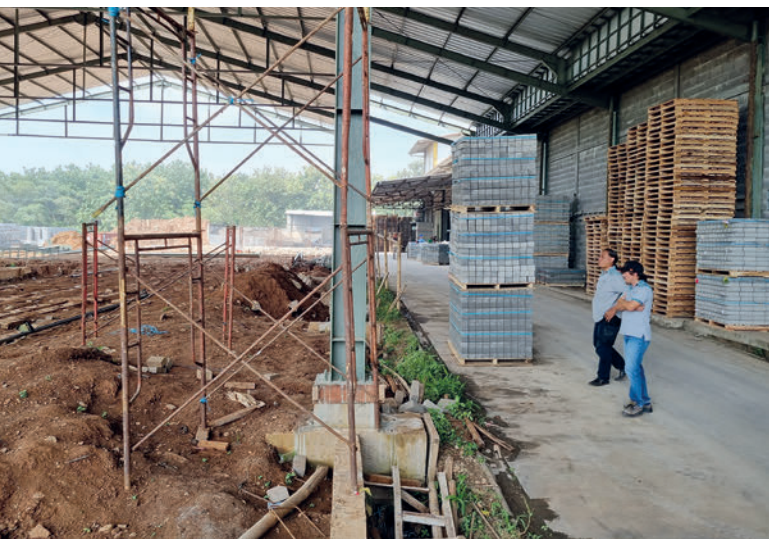
Foundation work for the new concrete block and paver line. On the right is the hall of the Hess RH 1500-3 concrete block and paver machine, purchased in 2010.
