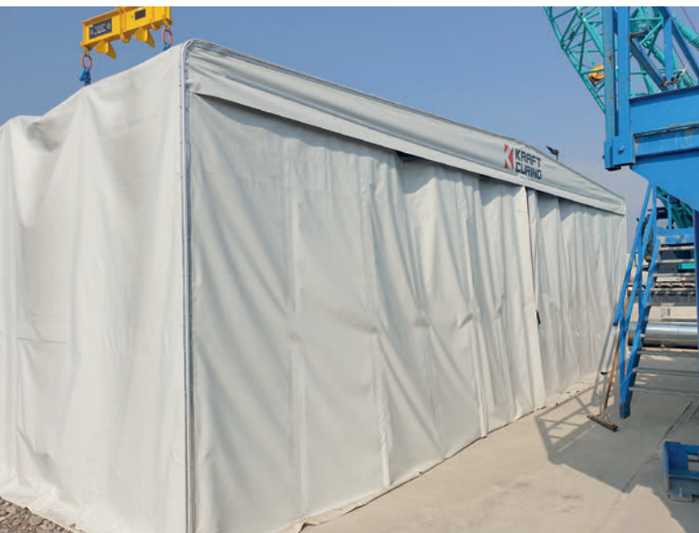
One of the five retractable curing enclosures (tents) initially supplied to the outdoor temporary casting area. The tents could be quickly dismantled and moved to the permanent facility once completed. A further ten tents were supplied as part of phase 2 delivery.
