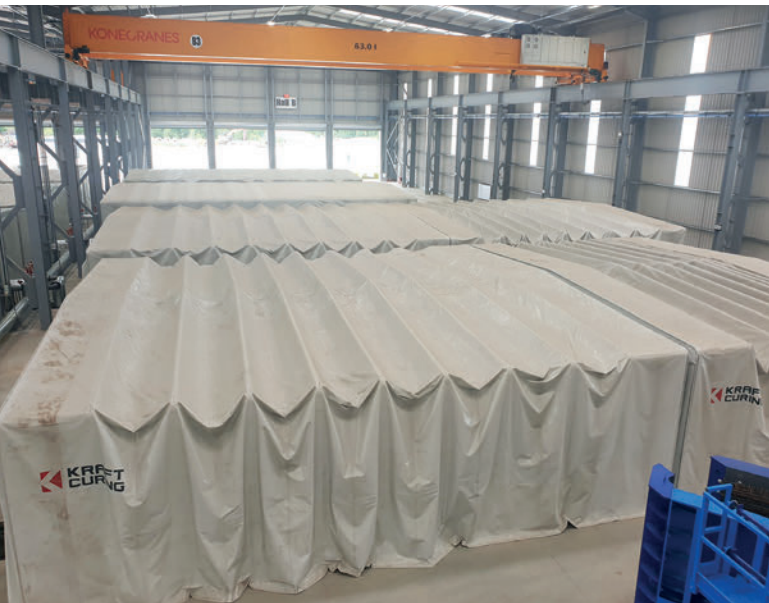
Some of the many retractable enclosures inside the secondary curing area. Each enclosure is capable of containing two concrete elements.
