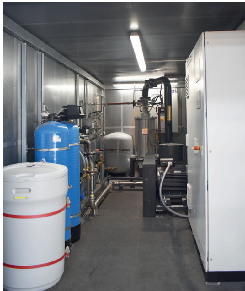
The Containerized Vapor Curing Unit with Water Treatment System.
