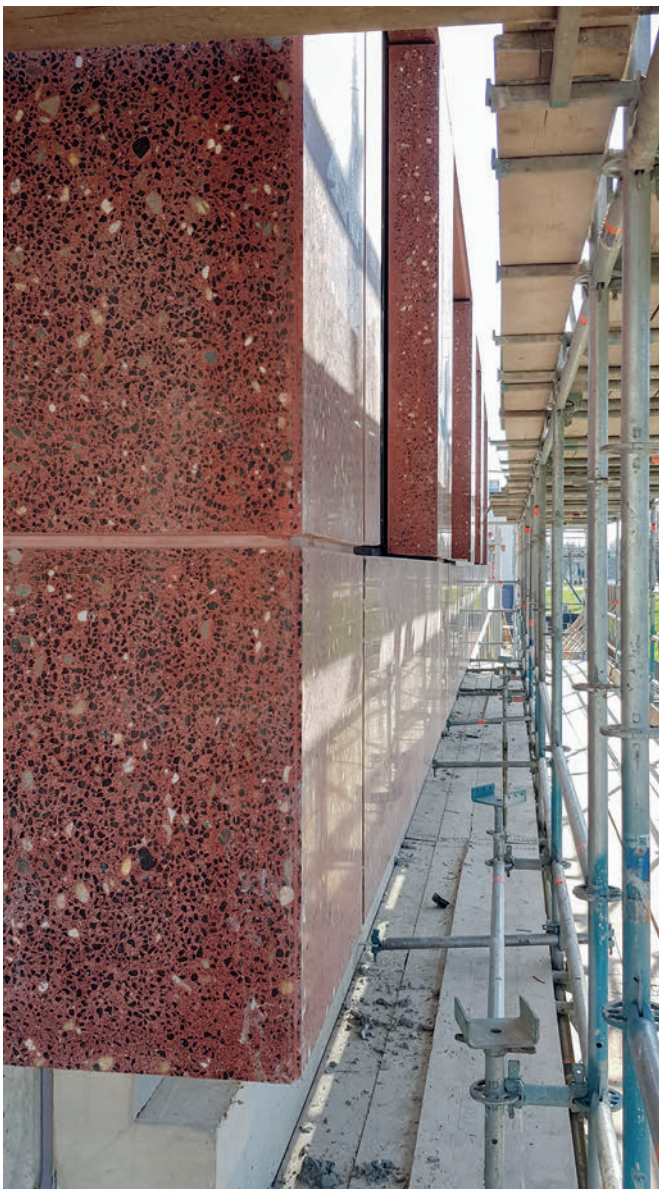
Facade elements by Preco at the construction of the hotel "The bridge" in Amsterdam.
