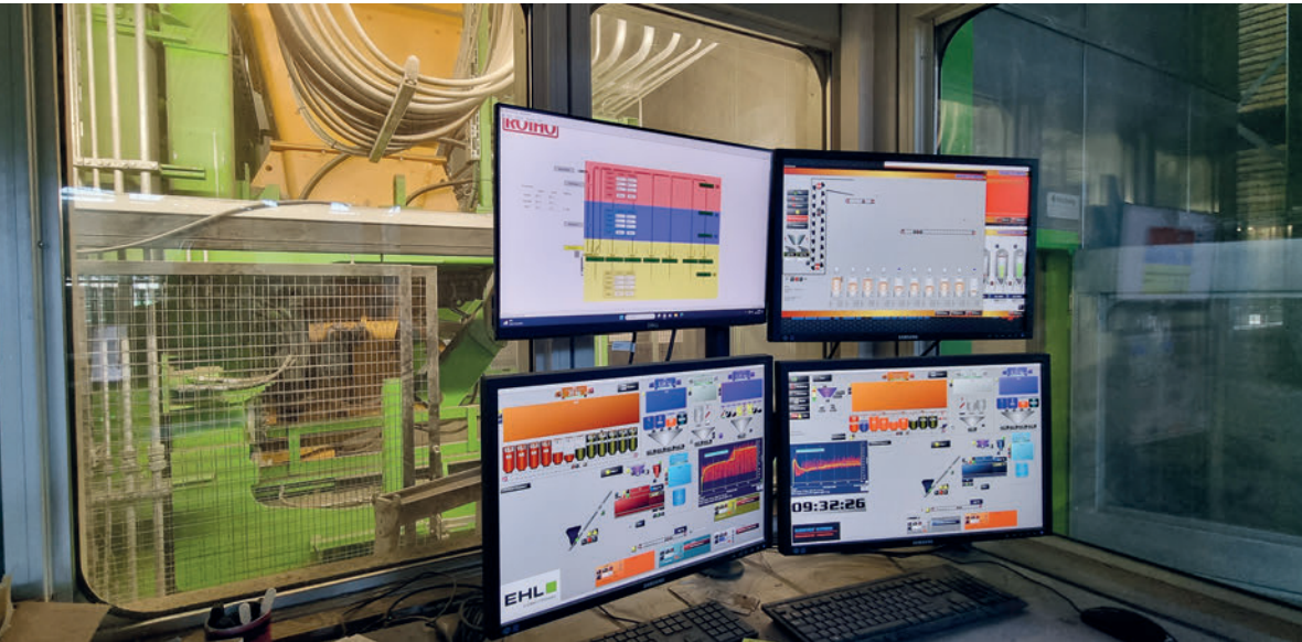
Centralised control of the dosing and mixing plant via the Sauter s-mix process control system.
