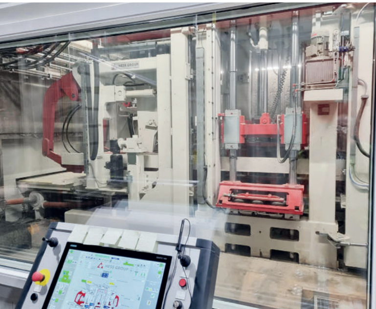
Control station & RH 2000-4 MVA (Hengelo)
