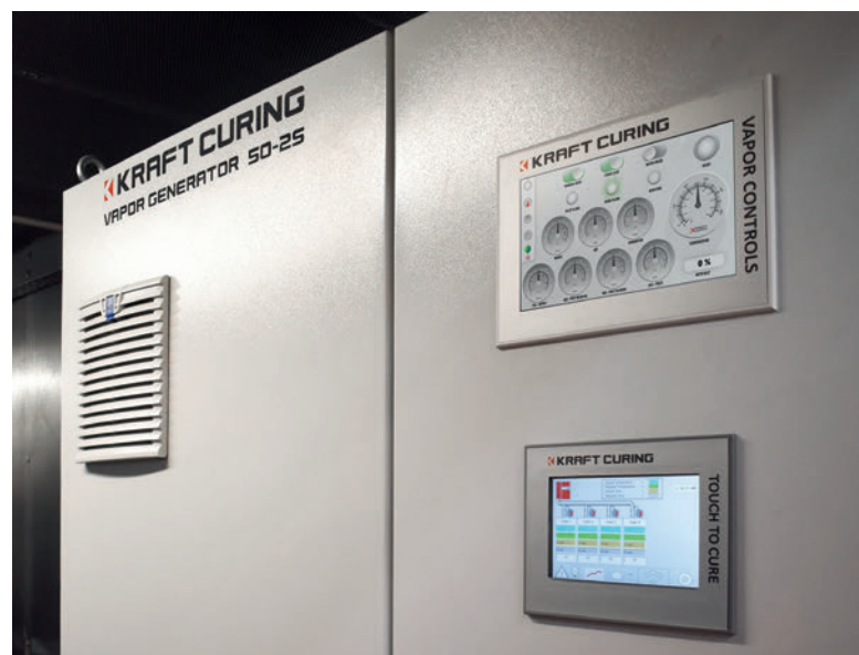
The Vapor Controls touchpanel (top-right) along with the AutoCure touchpanel (bottom-right) on the control cabinet in the containerized unit.
