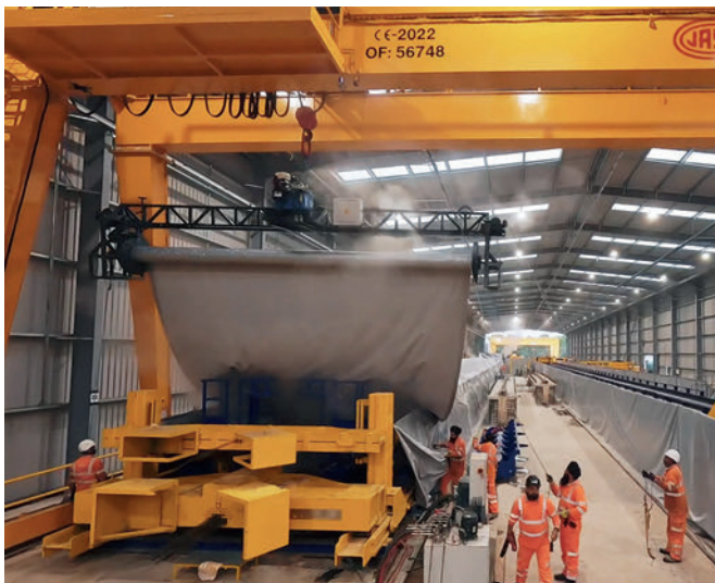
The motorized tarp roller moves along the form by way of the overhead crane, evenly unrolling the curing tarp.
