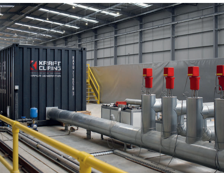
The Containerized Vapor Curing Unit along with 4 automatic vapor valves.
