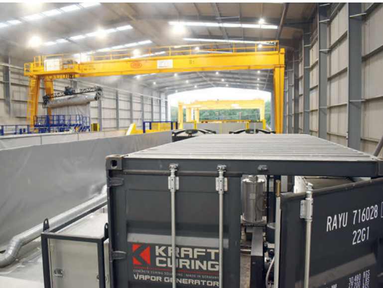
The decision was made by the FTB venture to invest in the Kraft containerized Vapor Generator
