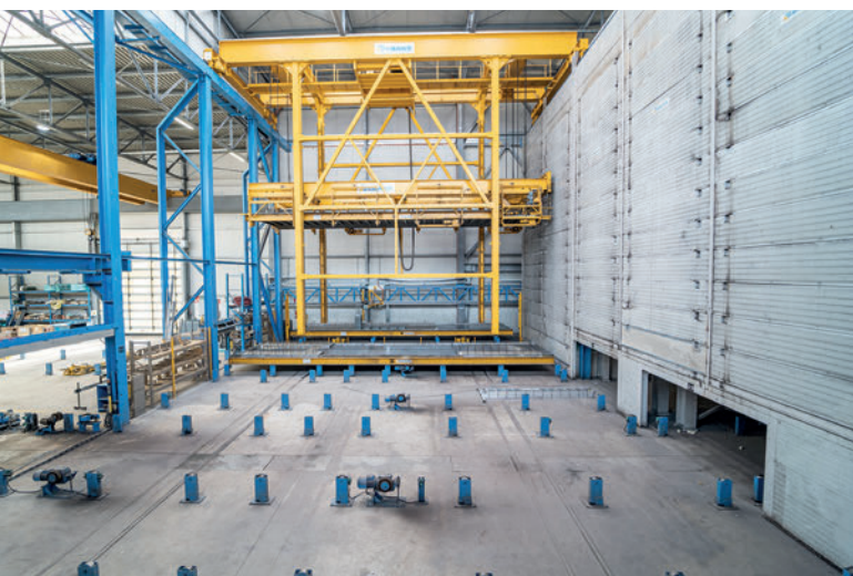
The automatic control unit transports the elements for effective curing, supported by the Green Code Curing Control.
