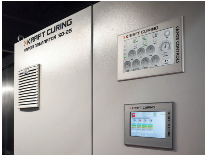
The Vapor Controls touchpanel (top-right) along with the AutoCure touchpanel (bottom-right) on the control cabinet in the containerized unit.
