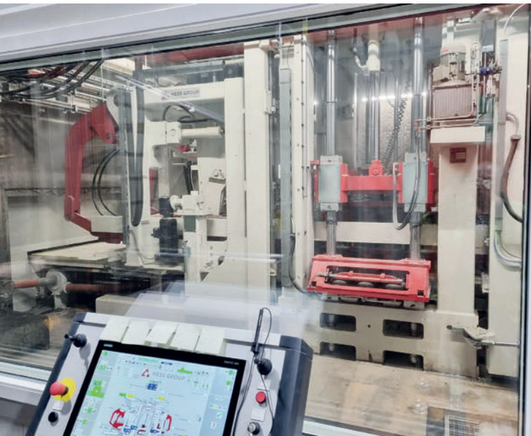
Control station & RH 2000-4 MVA (Hengelo)
