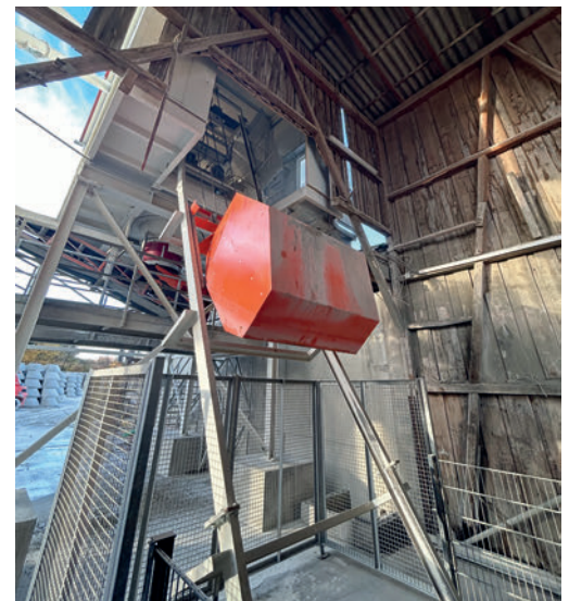
Feeder lift with fall protection
