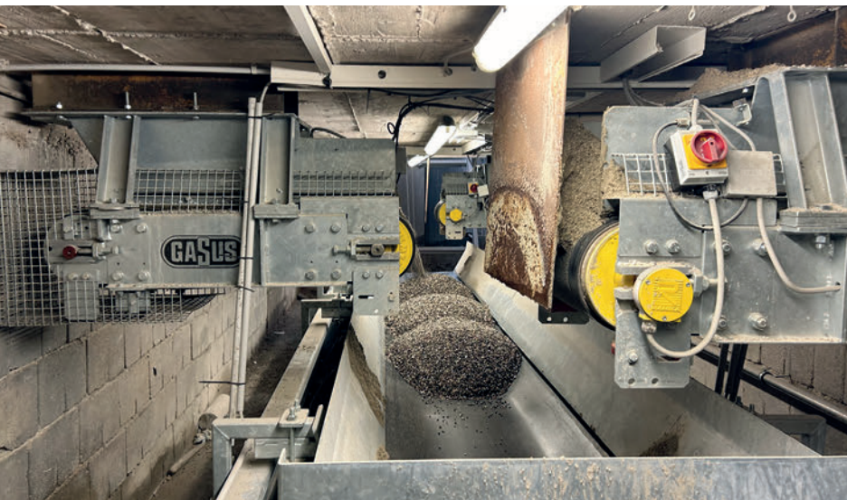
The dosing belts under the individual aggregate silos from the stockpile dose onto the new weighing belt.
