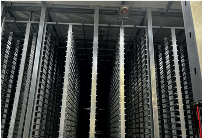
Curing Racks are in a single room to maintain temperature and moisture control for optimum product curing.
