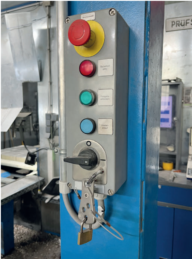
Safe and practical: Lockout-Tagout maintenance protection
