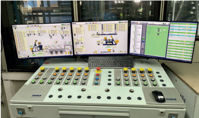
Control stand at Rünz & Hoffend before and after modernisation
