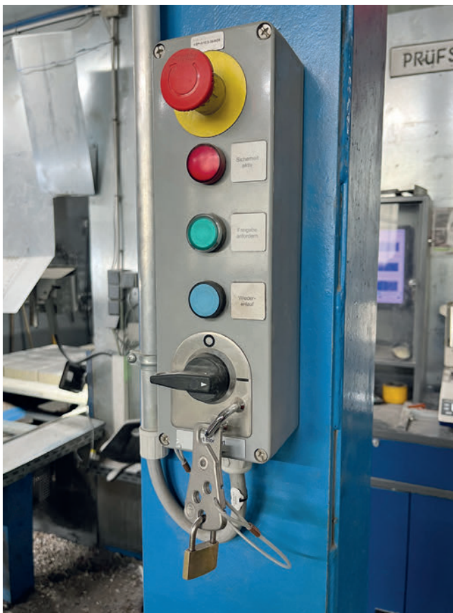
Safe and practical: Lockout-Tagout maintenance protection
