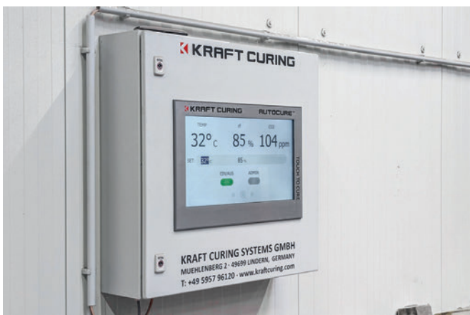
AutoCure® Accelerated Concrete curing chamber control screen
