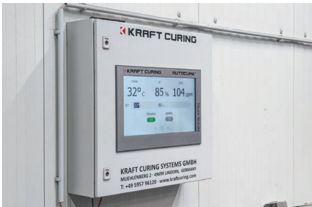
AutoCure® Accelerated Concrete curing chamber control screen
