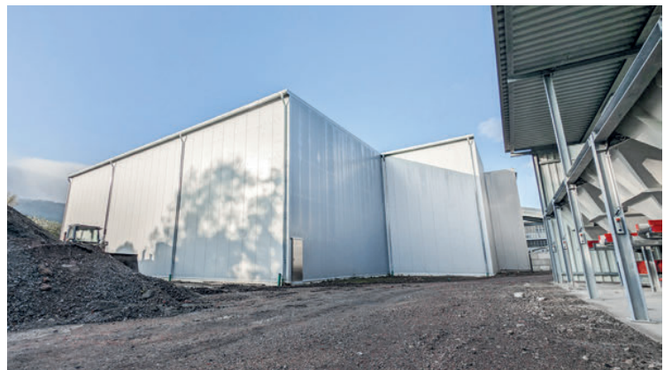
Curing chamber as a free-standing building and stainless steel escape door
