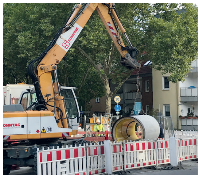
Datteln project: Lifting into the starting pit, piping detail with bentonite lubrication.
