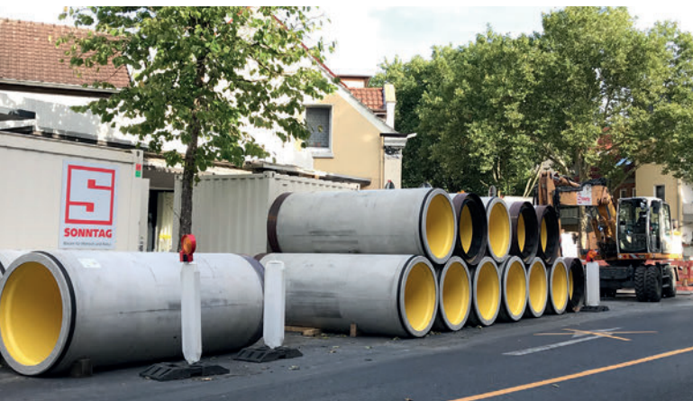
Datteln project, North Rhine-Westphalia, Germany: Site warehouse for DN 1200 Perfect jacking pipes from Beton Müller.
