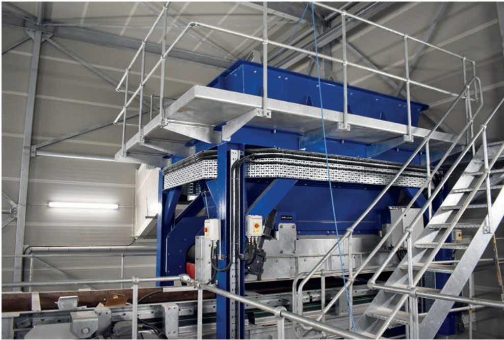
The Columbia Model 1600 block machine sits in the sound-insulated machine room.
