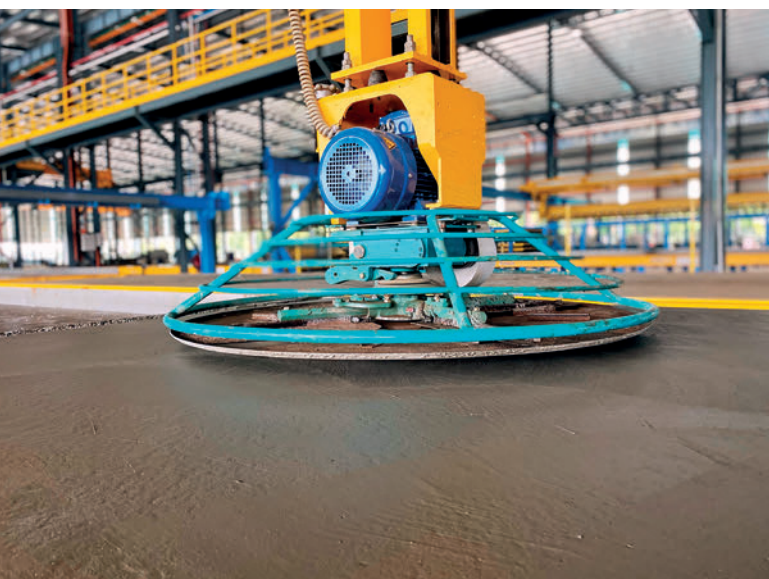
Effortless Finishing: Power trowel creates smooth surfaces, eliminating the need for painting.
