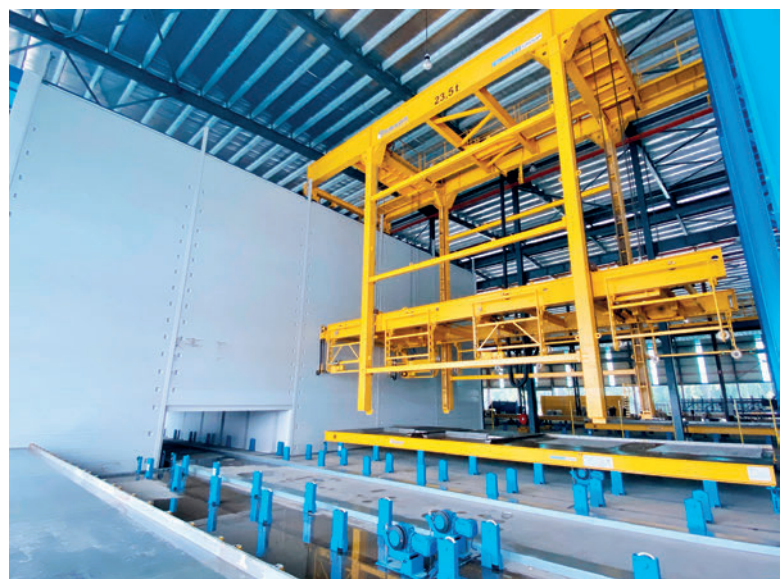
Efficient and automated storage system ensures fast and smooth factory operations.
