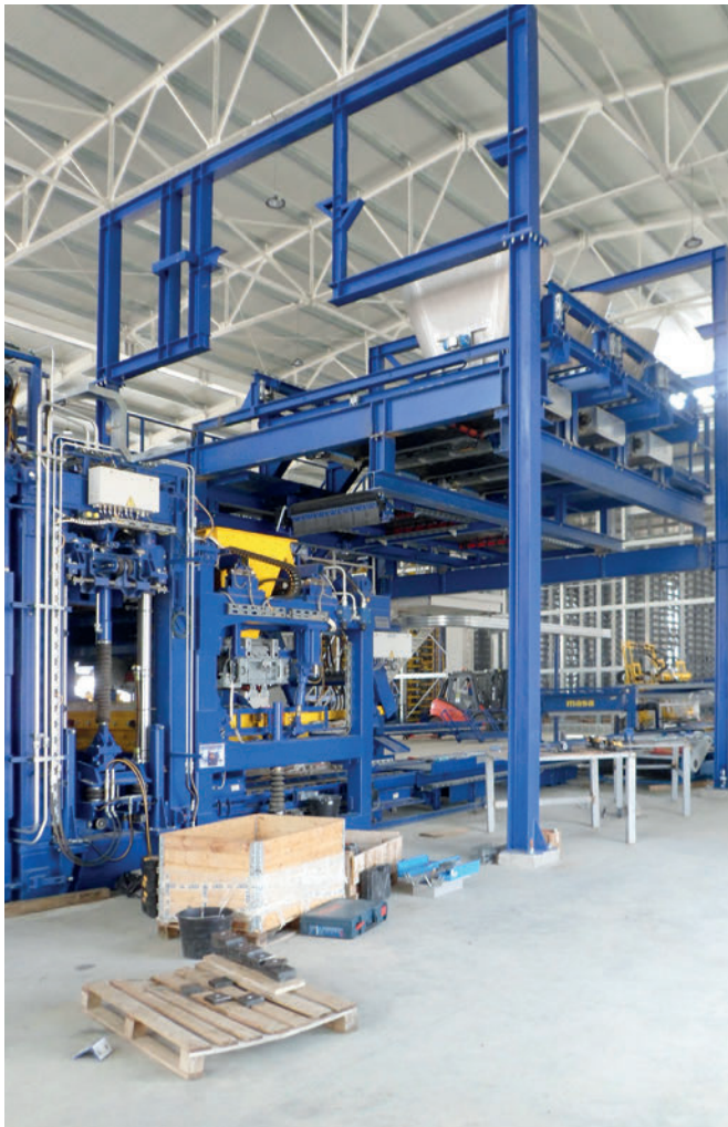
The assembly of the actual heart of the production plant, the Masa XL-R with Multi colour system (here for face mix concrete) required some routine and sensitivity.
