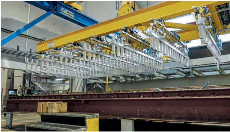
The installation of the new automated system was carried out during ongoing production and convinces with a daily output of up to 300 m 2 .
