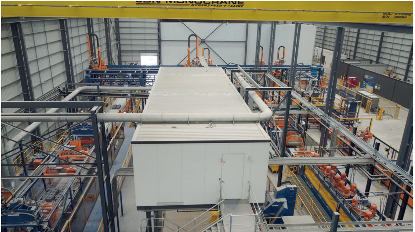
Top view of the value-adding line featuring pedestal for switch boards
