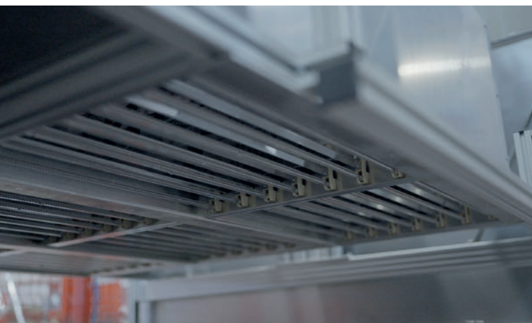
Coating line heating module
