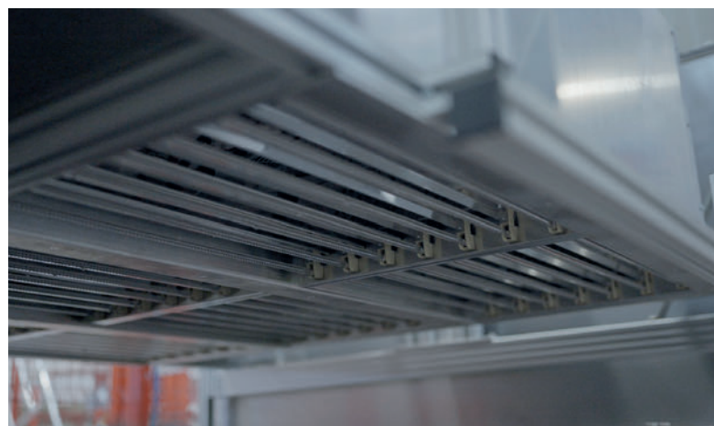
Coating line heating module
